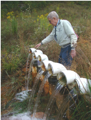
Thurman Korns, SCRIIP treasurer checks out discharge pipes at Wells Creek No. 7 AMD Treatment System
