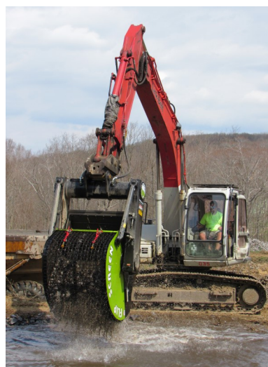
Limestone rock being washed and cleaned for reuse in Oven Run site E. Photo by Len Lichvar
