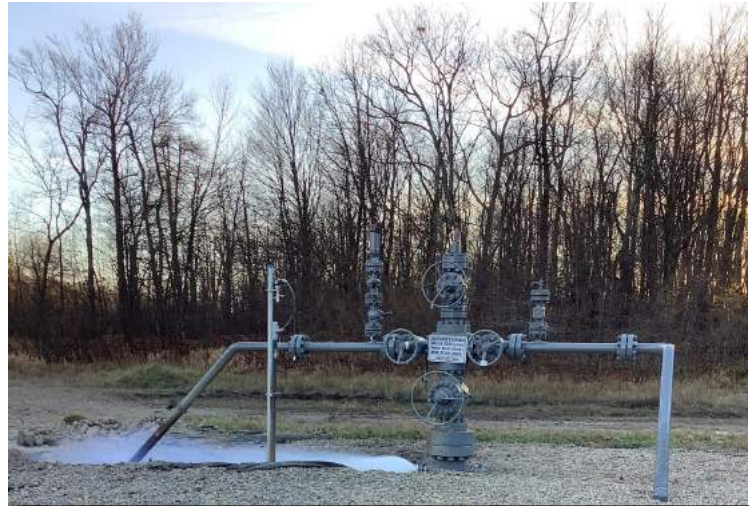
Gas Leak at Rager Mountain storage facility owned by Equitrans Midstream in Cambria County.
