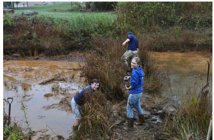
Engineering students CJ West, Ryan Fife, and Grace Bailey reconstructing a baffle between ponds.
