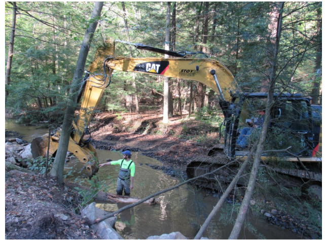
Somerset Conservation District Watershed Specialist, Greg Shustrick, directs stream improvement construction on the South Fork of Bens Creek. Photo by Len Liebvar
