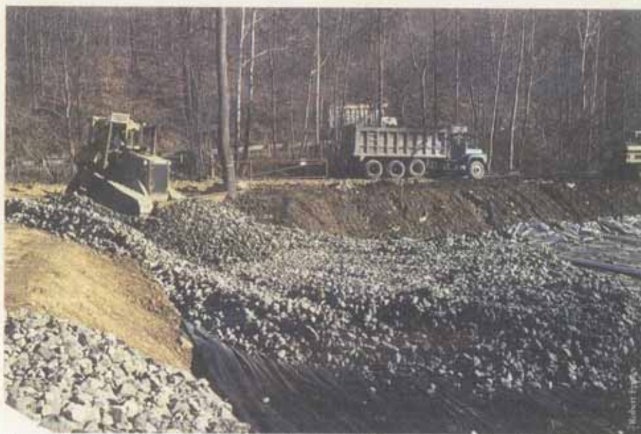
Heavy equipment moves stone during the construction phase of a vertical flow system along the lower Yellow Creek on state game lands near Indiana.
